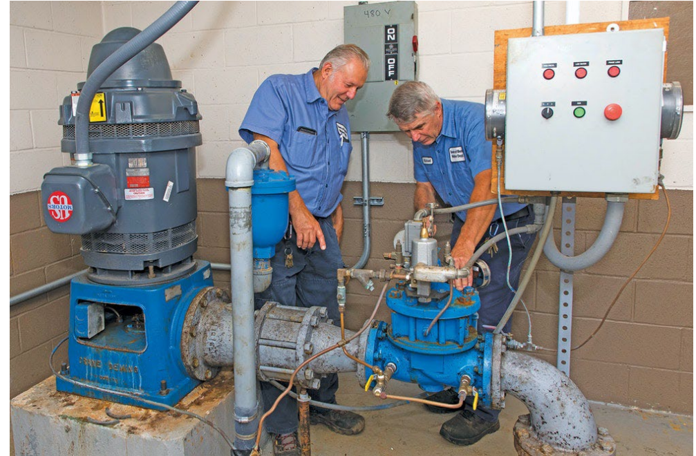
Elton Road Well Pump, Source: Municipal Sewer and Water Magazine
